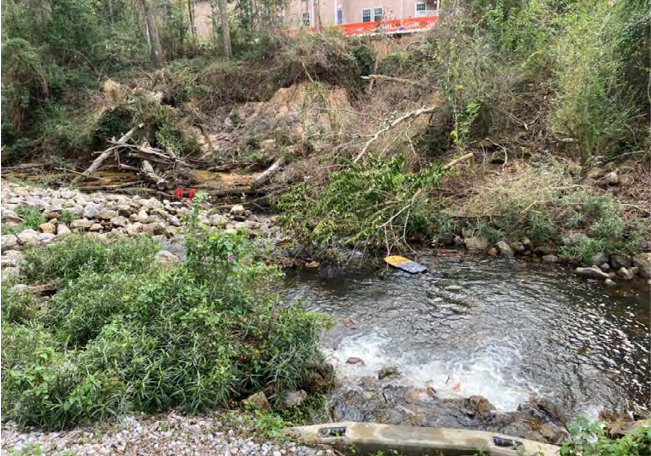
Learning from the Bank Erosion Downstream of Davis Highway
